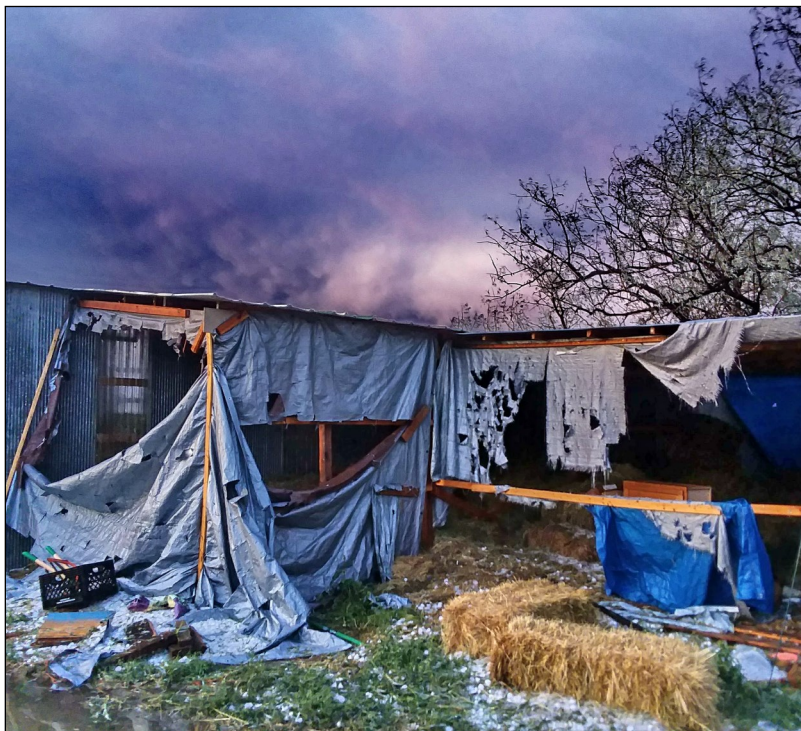
Straight-line winds and tennis ball-size hail did significant damage in Shepherd in August. At least 45 homes were significantly impacted including 15 that were no longer livable.
