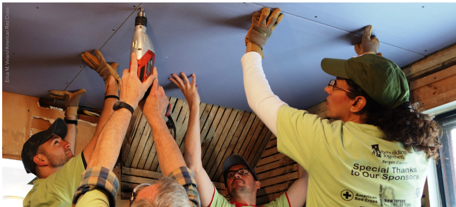
Red Crossers hang drywall at a Bergen County, N.J., home damaged by Superstorm Sandy, as part of Rebuilding Together's National Rebuilding Month.
